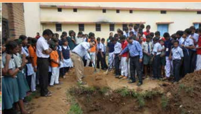
Water conservation - Soak pit in school.
